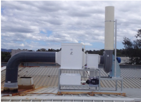
Roof mounted Advanced Air® fume scrubber 1200L/s.
